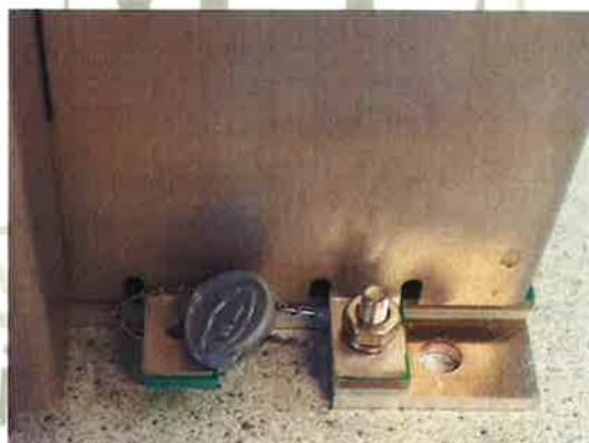
Sealing of the rack mounted transmitter
